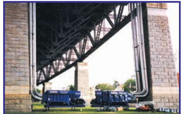
Mobile Dust Collectors installed on the Sydney Harbour Bridge to ventilate a large containment platform during Maintenance Blasting operations.
